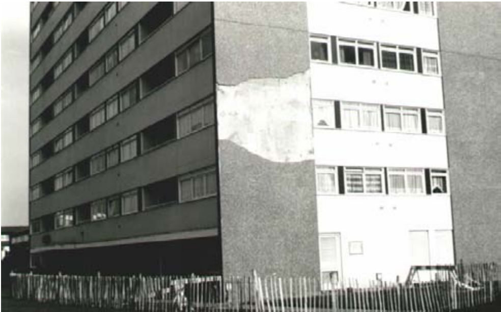
...after a block of external cladding fell off the outside of one tower block
