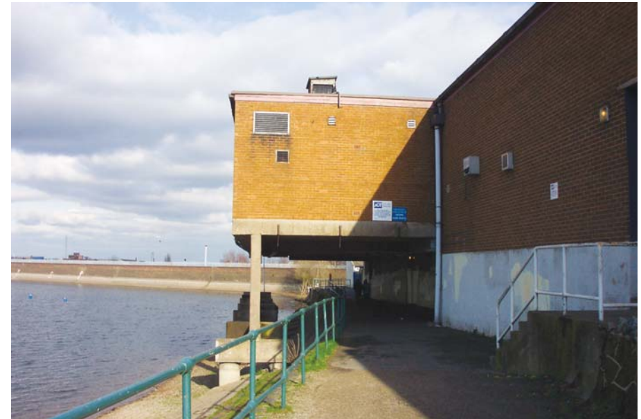
Community safety issues and poor quality design of existing Tower Ballroom
