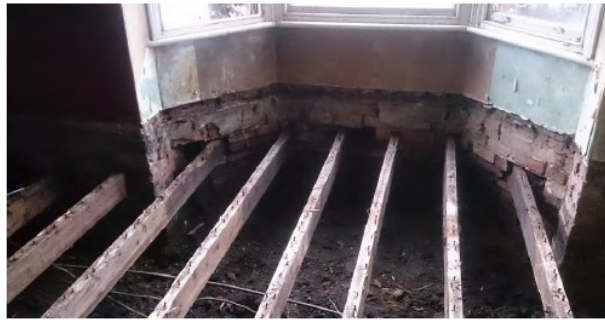
Achieving airtightness is possible in retrofit, but it is often necessary to strip back to the basic structure and perform basic repair work before methodically applying airtightness products and principles. Always consider risk of moisture and condensation. (Source: Eightpans)
