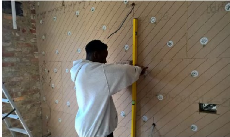
Installation of wood fibre insulation boards internally (Sources Back to Earth & ASBP)
