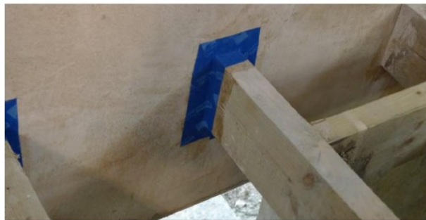
Applying airtightness tape to joist ends is a common measure required to achieve good airtightness in existing buildings. Large gaps may need filling with mortar first, and remember to apply a suitable primer. (Source: Ecomerchant)
