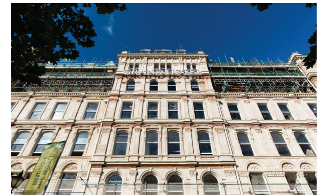
Restoration of the Grand Hotel, supported by the LEP's Growing Places Fund.
