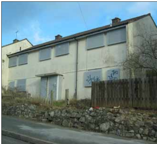
Examples of poor quality housing in the area
