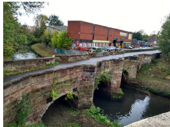
B - Perry Bridge is Grade 2 listed and a Scheduled Monument - known locally as the 'zig zag' bridge – it has medieval origins
