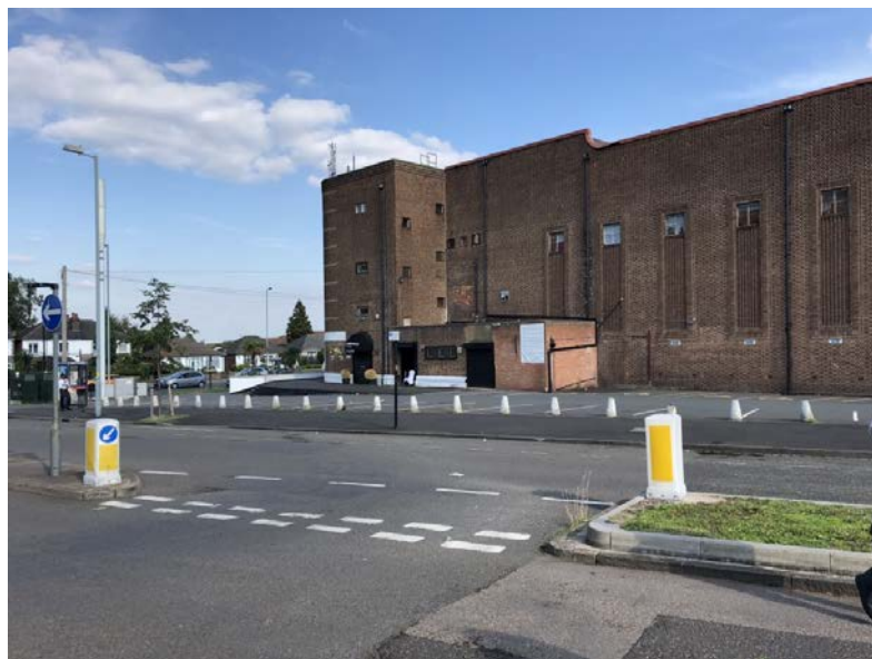
This landmark art deco building is prominent but the site treatment (bollards and tarmac) do not enhance the wider public realm or the setting of the listed building.
