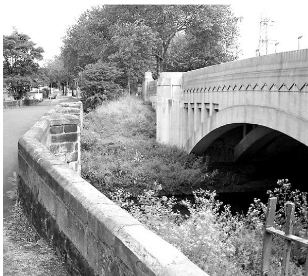
Perry Bridge (Grade II listed structure and Scheduled Ancient Monument) and 1930's bridge over River Tame.
